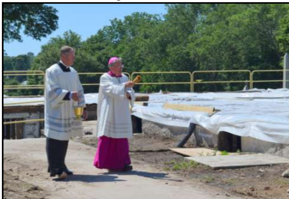
Bishop Cote and Father Perkins bless the foundation and site to prepare for the reconstruction of the church (blessing on page 6).
